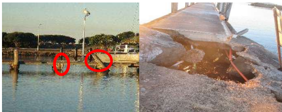
Figure 1 Damage at Crowdy Head harbour jetties due to seiche activity during the June 2016 storm [1]
